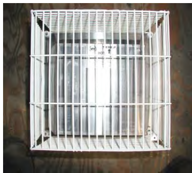
VIEW OF SAFETY CAGE
